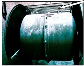
Interlocked guard on revolving drum
